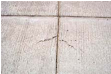
Figure 1: Upside-down smile ... Typical smiley-face cracking is shown at left. Illustration is from the driving lane looking toward shoulder.
