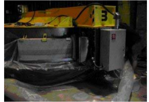
Figure 4 – The grinding unit with dust collection system in place
