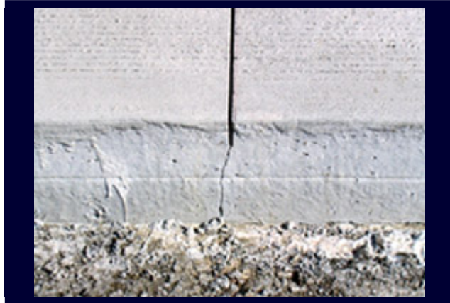
Joints control natural cracking when design and constructed properly.
