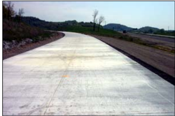
The concrete pavement work on SR-840, Williamson County, Tenn., was done by Interstate Concrete Constructors, LLC.
