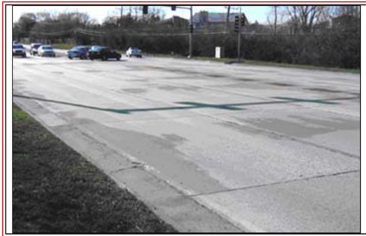
An inadequate understanding of the state specification left this project with 30% holidays.
