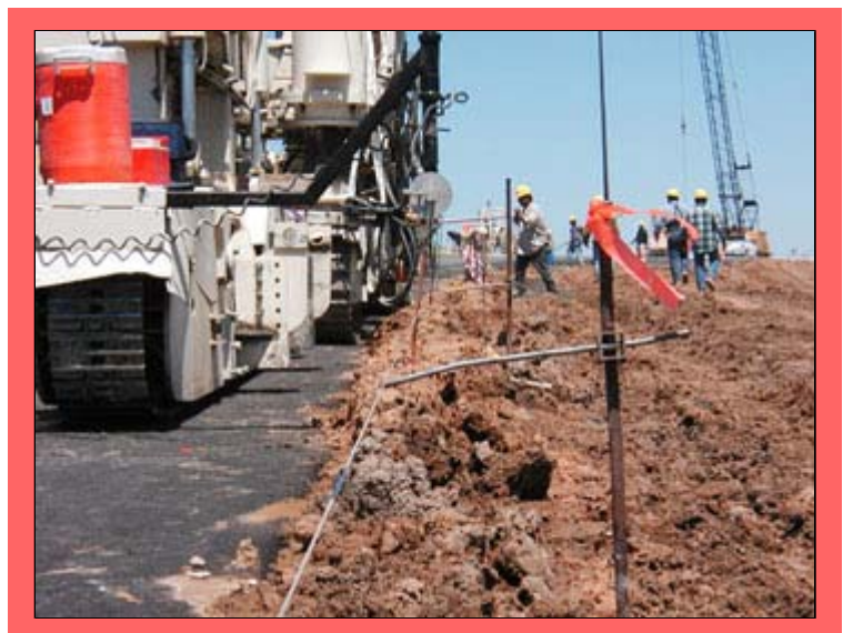
To increase the visibility, some contractors tie brightly colored ribbons to the stringline. Personnel near the stringline should avoid touching the stringline.
