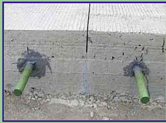
The key to saw cutting joints in pavements with dowel bars is doing it right the first time.
