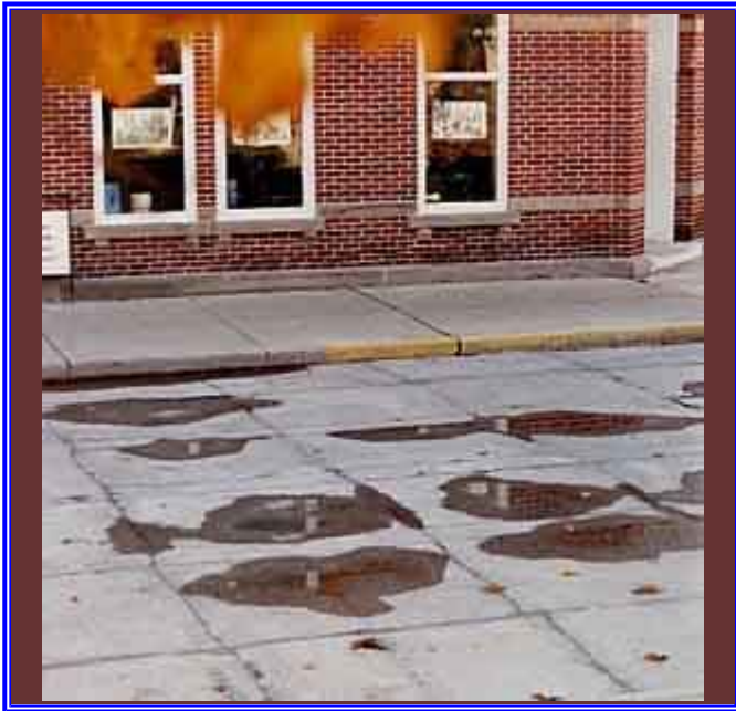
Knowing what to do about a rained-on concrete is the key to a long-lasting pavement, such as this 103-year-old street -- the nation's first portland cement concrete roadway in Bellefontaine, Ohio. (Photo courtesy: Ohio Ready Mixed Concrete Association)
