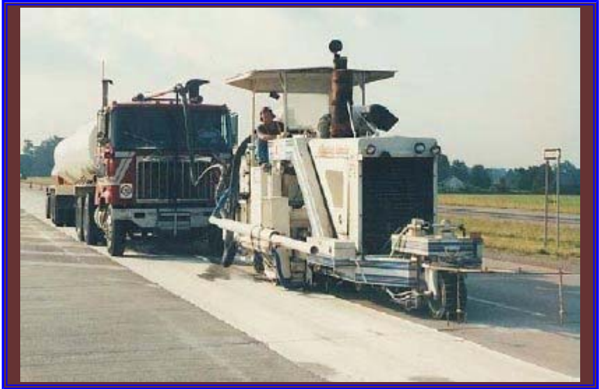
A diamond-grinding machine is used for removing the non-durable surface, re-texturing the pavement, and smoothing out the ride.
