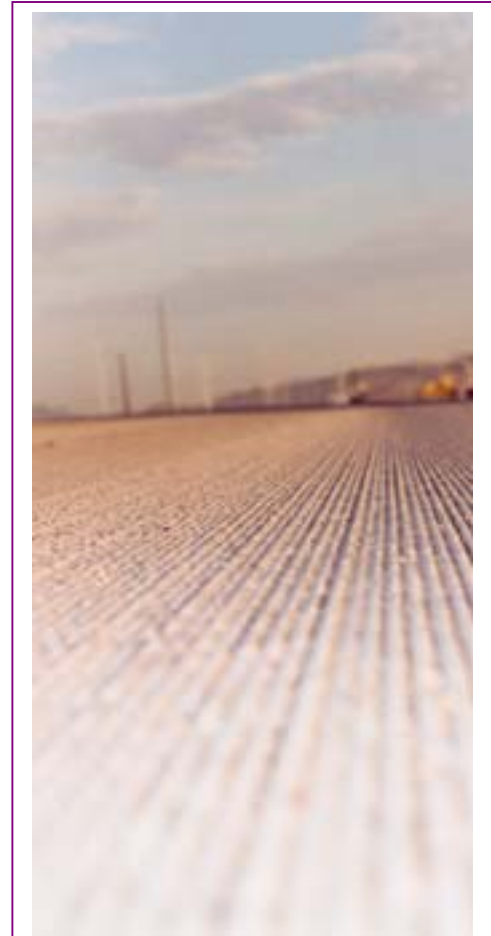
Research has shown that diamond ground concrete pavements are at least as quiet as asphalt pavements.
