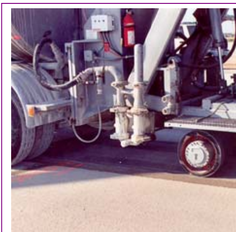
Operator diamond-grinds a section of concrete pavement used for tire/pavement noise testing in Arizona.
