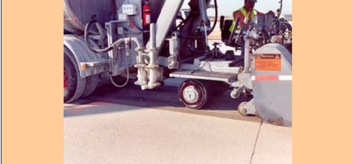
Photo depicts the diamond grinding of a concrete pavement. Research shows that diamond-ground pavements are at least as quiet as asphalt pavements. Diamond grinding restores pavement surfaces, removes joint faulting, and improves skid resistance
