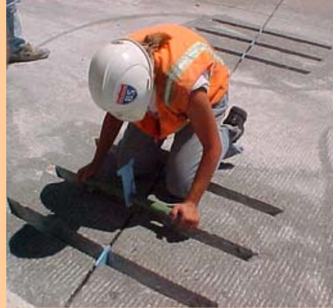
Worker installing retrofit dowel assembly into prepared slot. Note blue joint re-former placed in-line with existing joint. Dowel bar retrofit restores load transfer at undoweled transverse joints or cracks.
