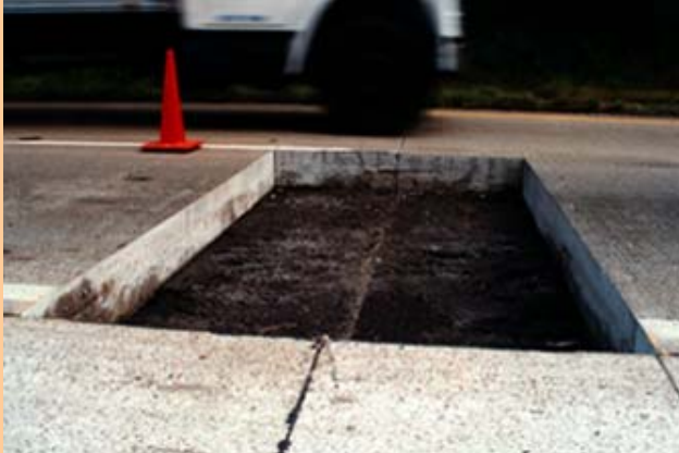
Photo depicts full-depth repair prior to drilling holes for dowels in adjacent slabs. Full-depth repairs address almost all structural distresses and will extend the original pavement design life.
