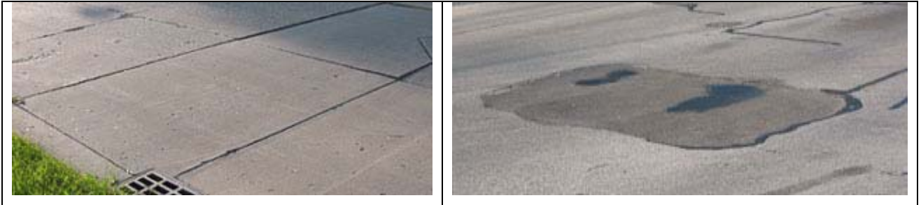
Photos depict utility cuts in concrete (L) and asphalt (R).
