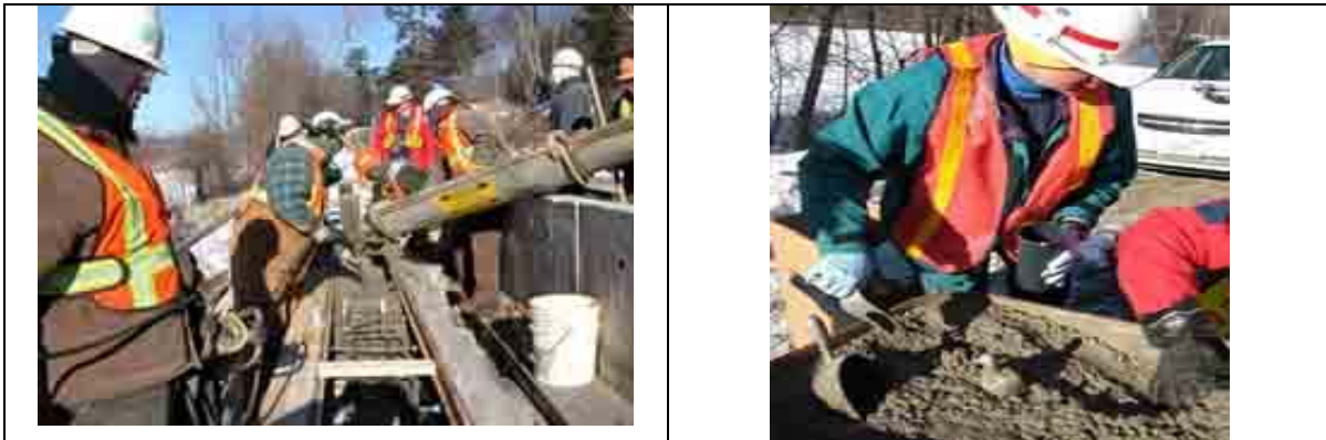
Workers place concrete in cold weather (left) and collect samples of the concrete mix for testing (right).
